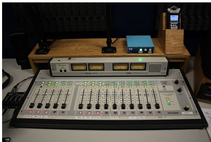
Fig. 2 Arrakis ARC 15 main console
